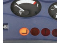
Lifting interlock lamp on the control panel
